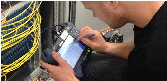
2019 Kitco Panel Project Fiber Optic Testing Enhancement for Cost Reduction
