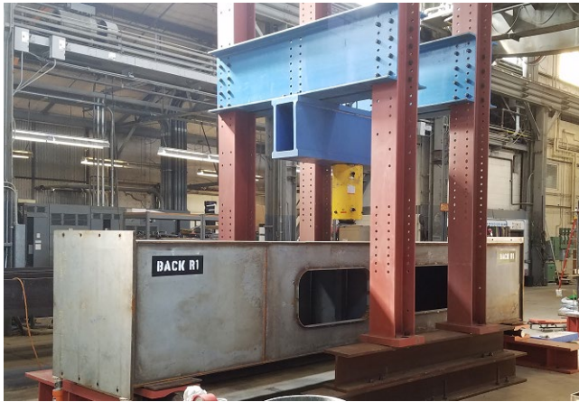
Simplifying Inner bottom construction by reducing parts and improving design to increase efficiencies
