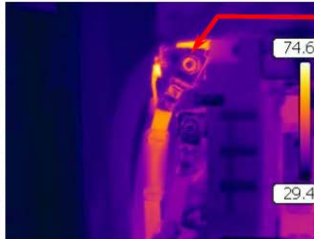
Before Repairs Thermogram
